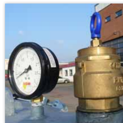
Pressure gauge and safety valve
