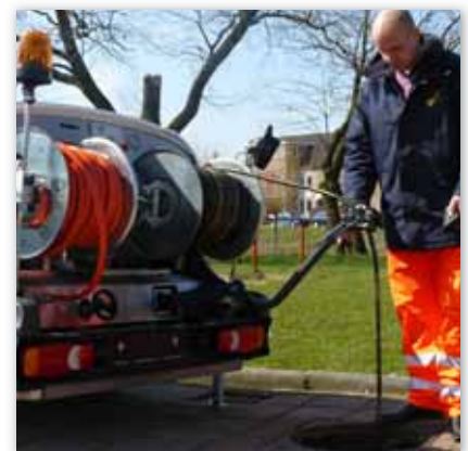
Control panel within reach of the HP reel; fitted at an ergonomic working height
